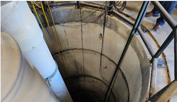
Underdrain Wet Well
