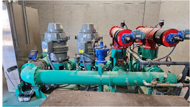
Irrigation Pump (Not accepted in this report)
