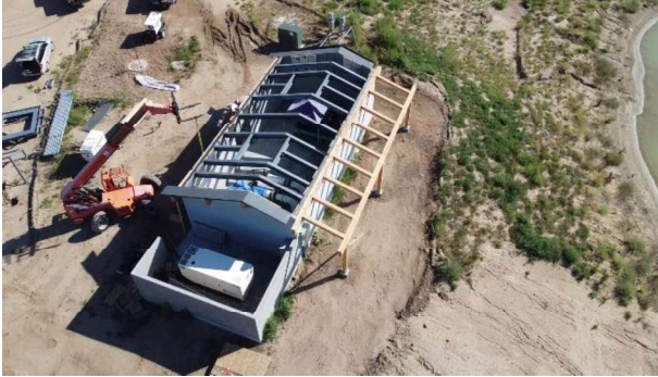
Tract C & Non-Potable Pumphouse View: North
